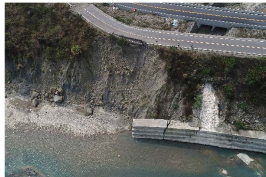
圖 1 水流淘刷造成近岸崩塌及道路坍方 Fig. 1. The near-bank landslides and road damage caused by flow scour.
