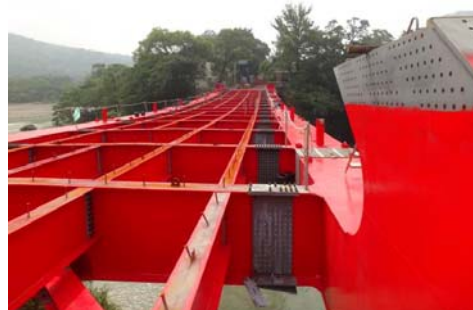
圖 3-7 高張力螺栓均未完成鎖緊及剪斷 Fig. 3-7 High tensile bolts locking and cut were completed
