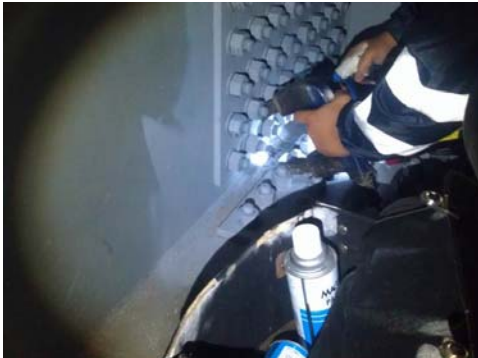
圖 3-10 磁粒檢測(MT)結果均未發現異常 Fig. 3-10 Magnetic particle testing (MT) results were not unusual
