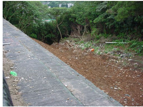
圖 8. 修復後坡腳無排水路並裸露 Figure 8. Repaired hill slope without proper drainage and vegetation cover.
